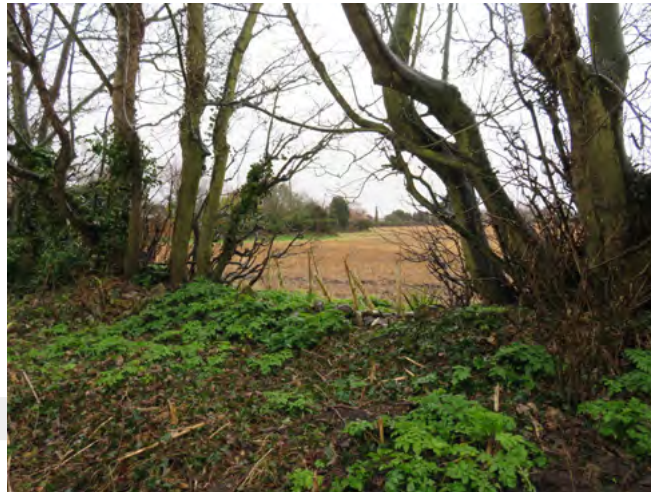
Collapsed flint wall along The Street
