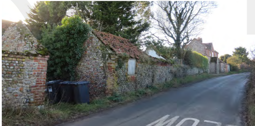
The outbuildings of Green Farm are in a very poor condition
