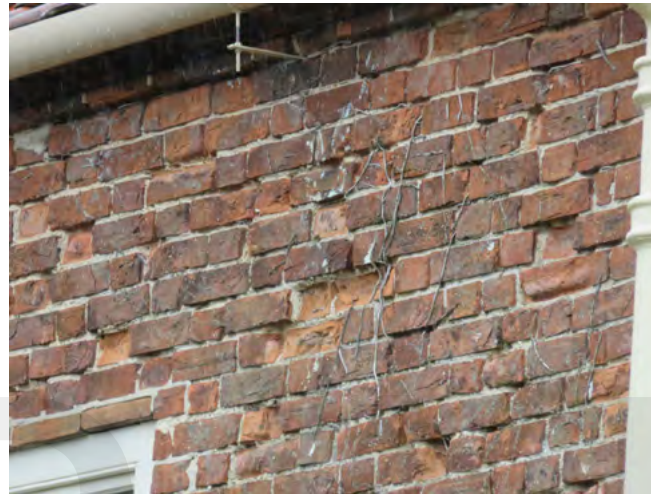
Norfolk bricks are typically soft and prone to erosion especially if the pointing is not maintained
