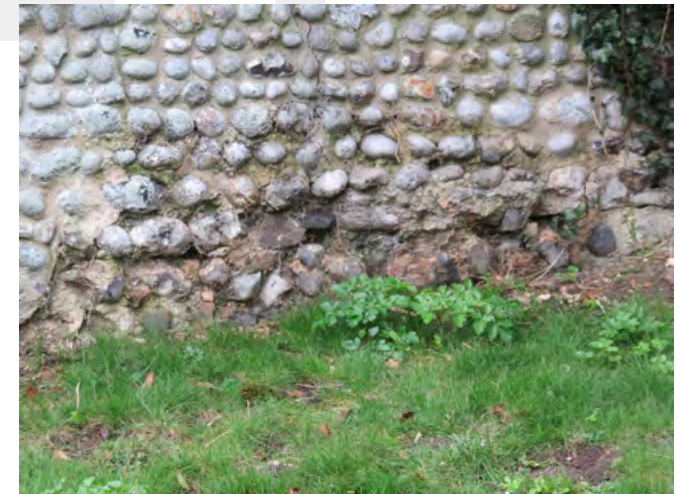
Failing flint wall on Leatherpool Lane
