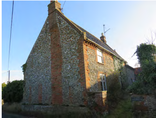
Green Farmhouse is a significant local landmark building but its condition detracts from its appearance and that of the Conservation Area
