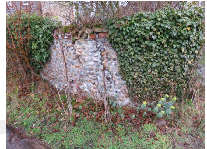
Damaged flint wall along The Street
