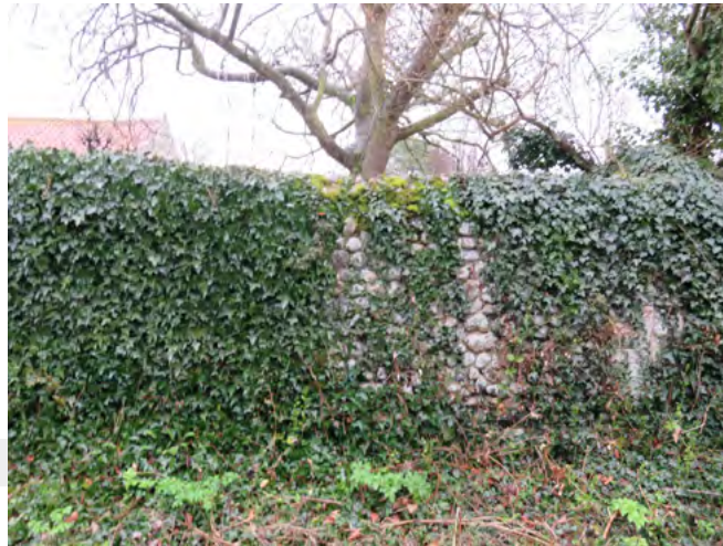
Ivy engulfed wall on Chapel Lane
