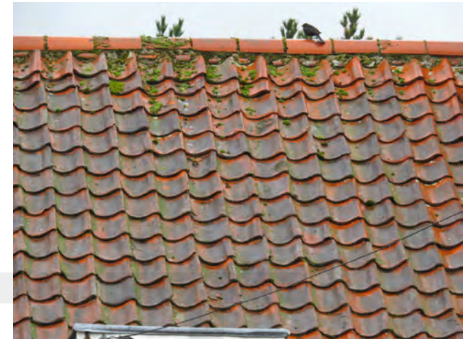
Moss on a roof affects the appearance of the building but also holds moisture against the tiles. The moss also blocks gutters and drains when it is dislodged
