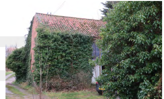
Ivy growth on the double height barn at Green Farm
