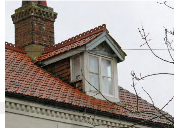
Dormer windows are particularly vulnerable and need to be regularly maintained
