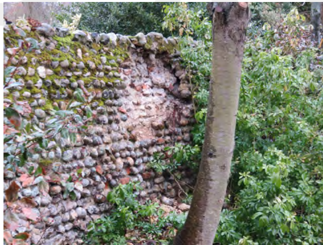
Failing flint wall on Chapel Lane
