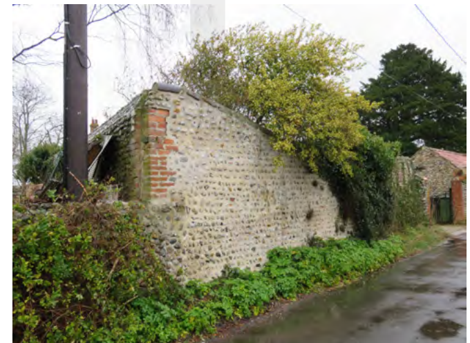
Excessive mortar alters the appearance of flint walls
