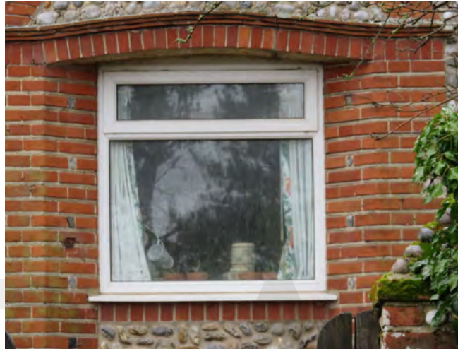
Example of an inappropriate uPVC window
