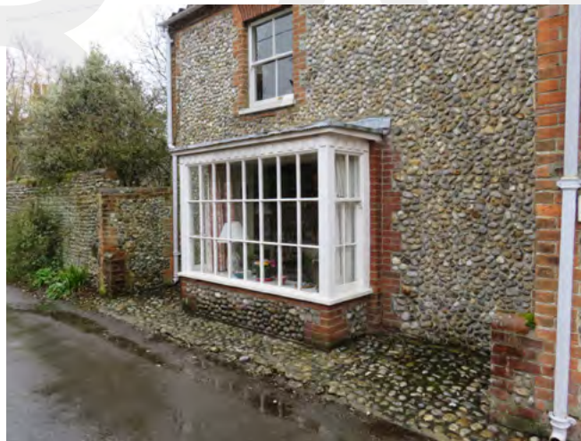
Cobbled floorscape on Chapel Lane is being damaged by vehicles
