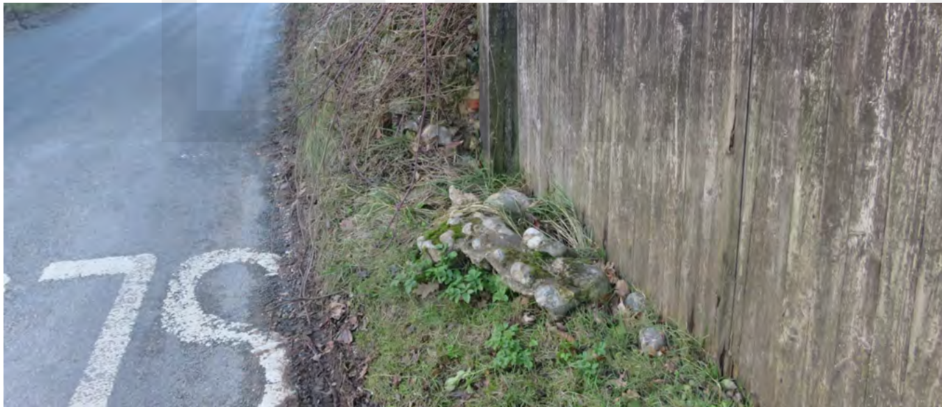
Engulfed and failing flint wall on Blakeney Road
