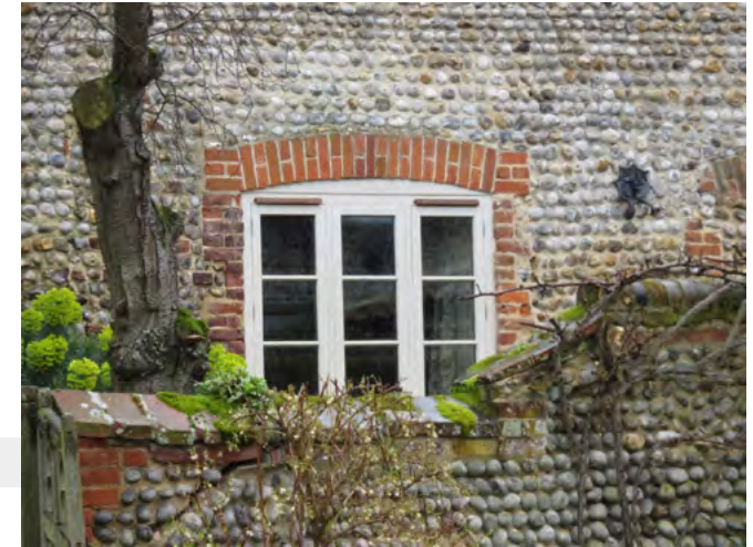
Window vents added to replacement windows detract from the appearance of the windows
